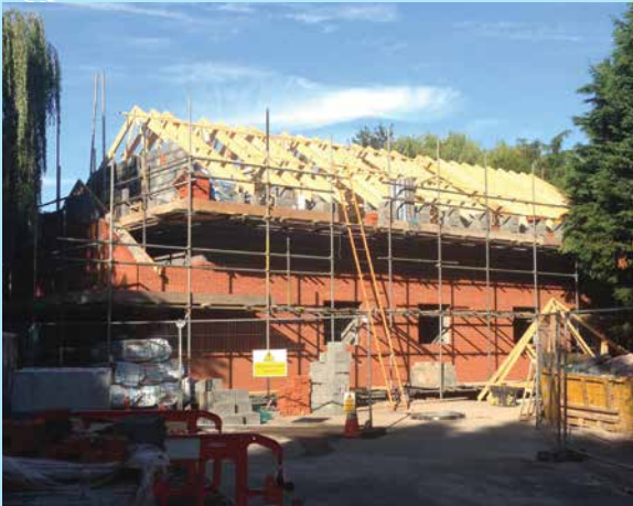
Building work is well under way at the Glenfield scheme in Leicestershire.
